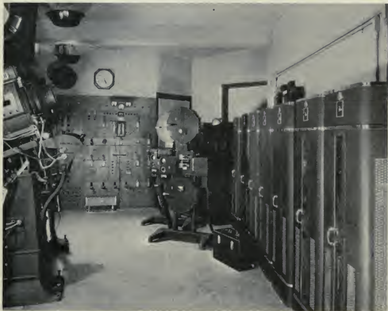
FIG. 2. Installation in the Carthay Circle Theater, Hollywood.
